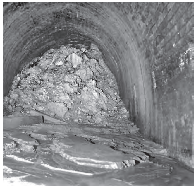
A total roof collapse which probably occurred in 1954 was found \frac{7}{8} mile from the California portal during a navigation of the Lapal Tunnel in 1961. Photo from Edwin Fasham, Lapal Canal Trust
